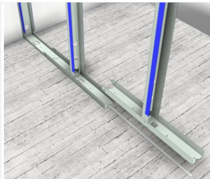
The JUUNOO Glue is applied to the center line of the wall on the floor.
